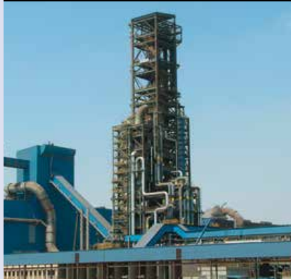
HOT TRANSPORT CONVEYOR (Distances < 200m)
