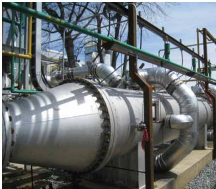
FIGURE 2 TRS® Demonstration Plant
