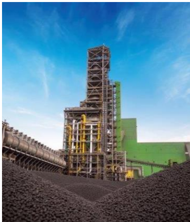
Photo: Tosyali Algerie, MIDREX CDRI/HDRI Plant Capacity: 2.5 mtpy, Location: Bethioua (Oran), Algeria
