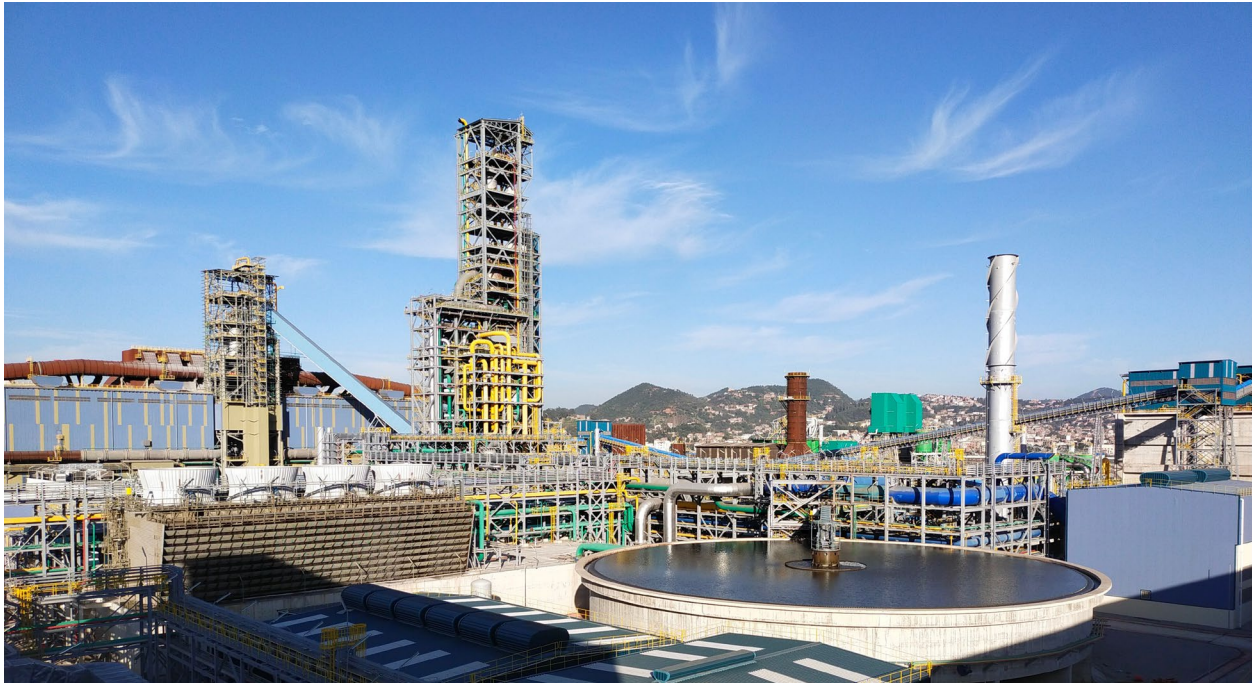
2.5 million t/y MIDREX Plant at AQS Bellara Steel Complex
