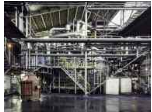
Figure 10 - ITmk3 ® Pilot Plant at Kakogawa Works
