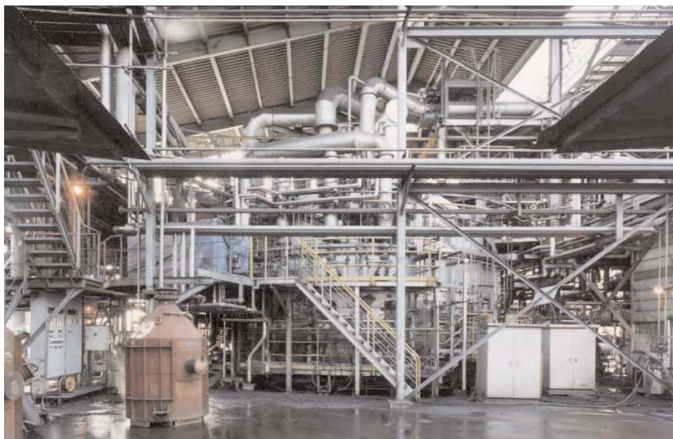
Kakogawa's FASTMET® waste recycling facility
