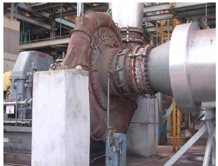
FIGURE 3 Centrifugal Compressor at LION
