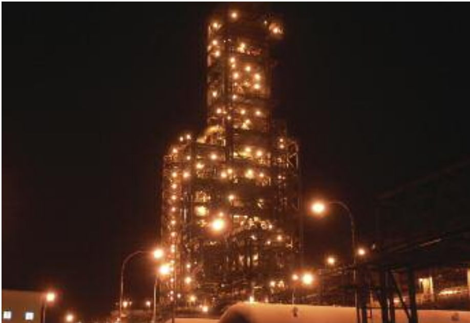
Figure 3 - Qatar Steel: View of DRI-2 MIDREX Plant at night
