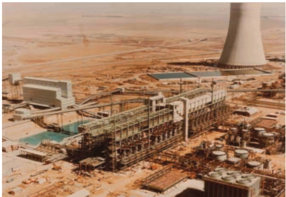
Battery of 40 MK IV Sasol-Lurgi Fixed Bed, Dry Bottom Gasifiers under Construction in South Africa (Circa 1980)
